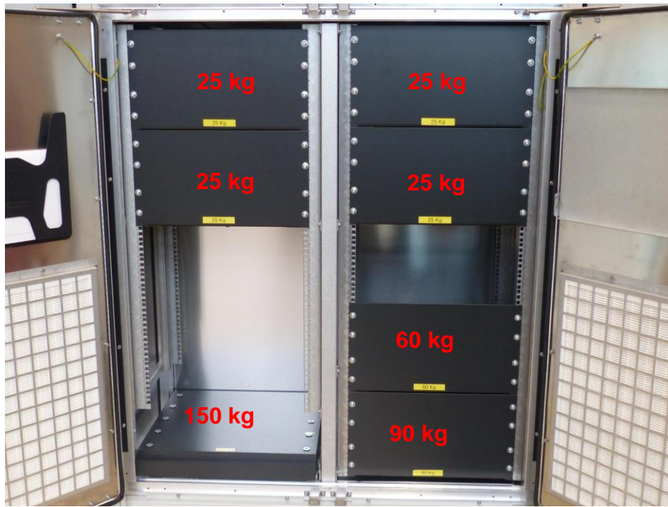
Photograph n°16 : Distribution of the ballasts inside the cabinet
