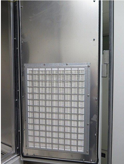
No dust inside the cabinet
