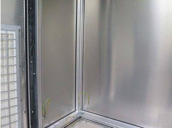
No dust inside the cabinet
