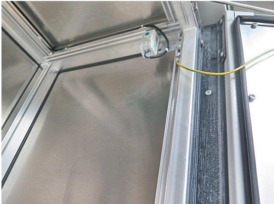
No dust inside the cabinet
