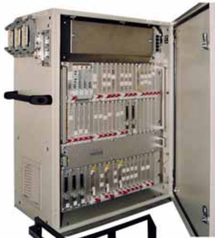
Application: Signalling control systems
