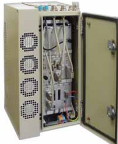
Application: Mobile telephony system
