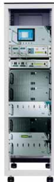
Application: Train control system
